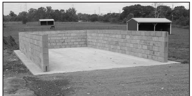
A well-drained manure storage structure is integral to a good waste management plan. This one was designed with the aid of the Natural Resources Conservation Service.
